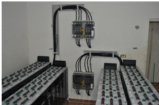
Battery Bank location
