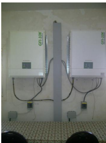
Voltage Controller/ Inverter & windsensor Datalogger in one housing
