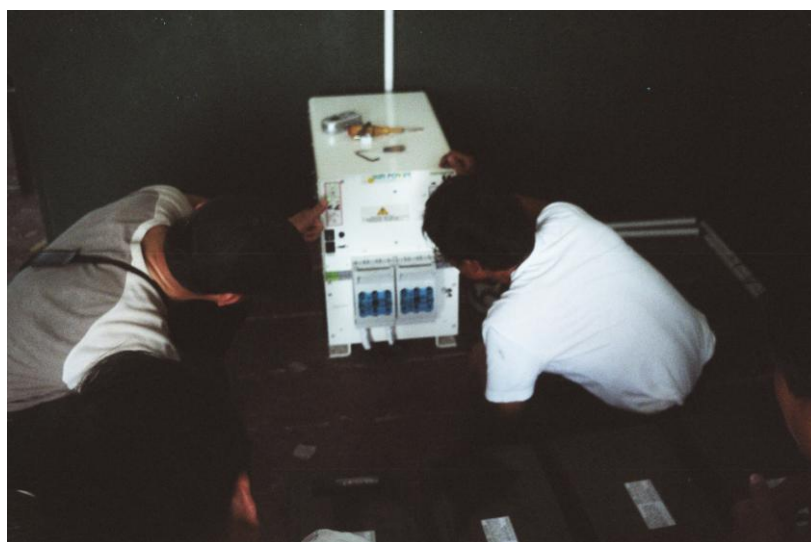
Installing “Sunpower” Hybrid Bydirectional inverter of 5 kW
